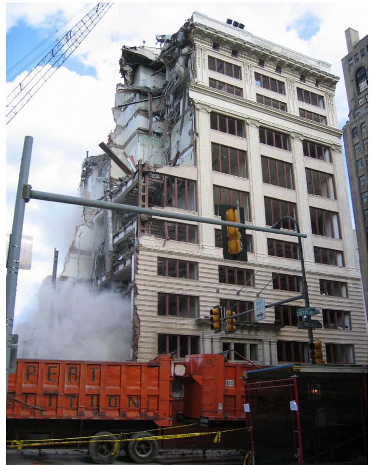
Demolition of Odd Fellows Temple, Broad & Cherry Streets, 2008, Photograph by Michael J. Seneca.
